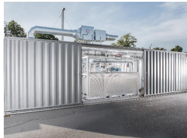
150 kW SOEC unit in Dresden, Germany
